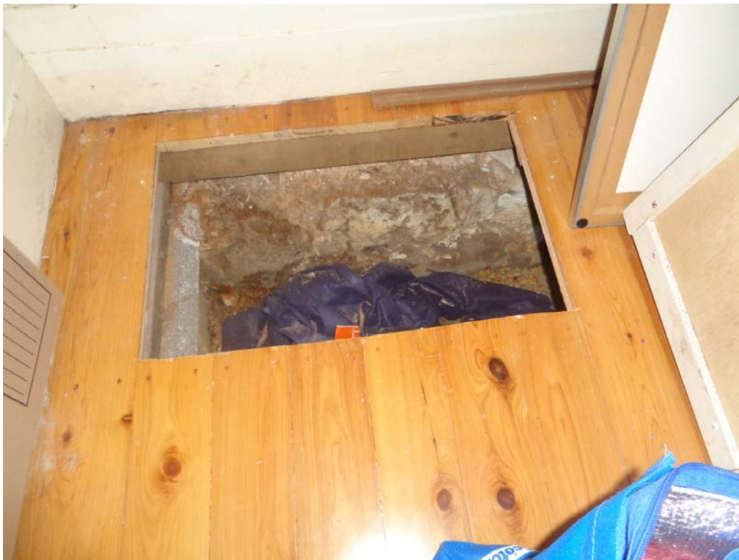
Sub floor access. Unable to gain full access
