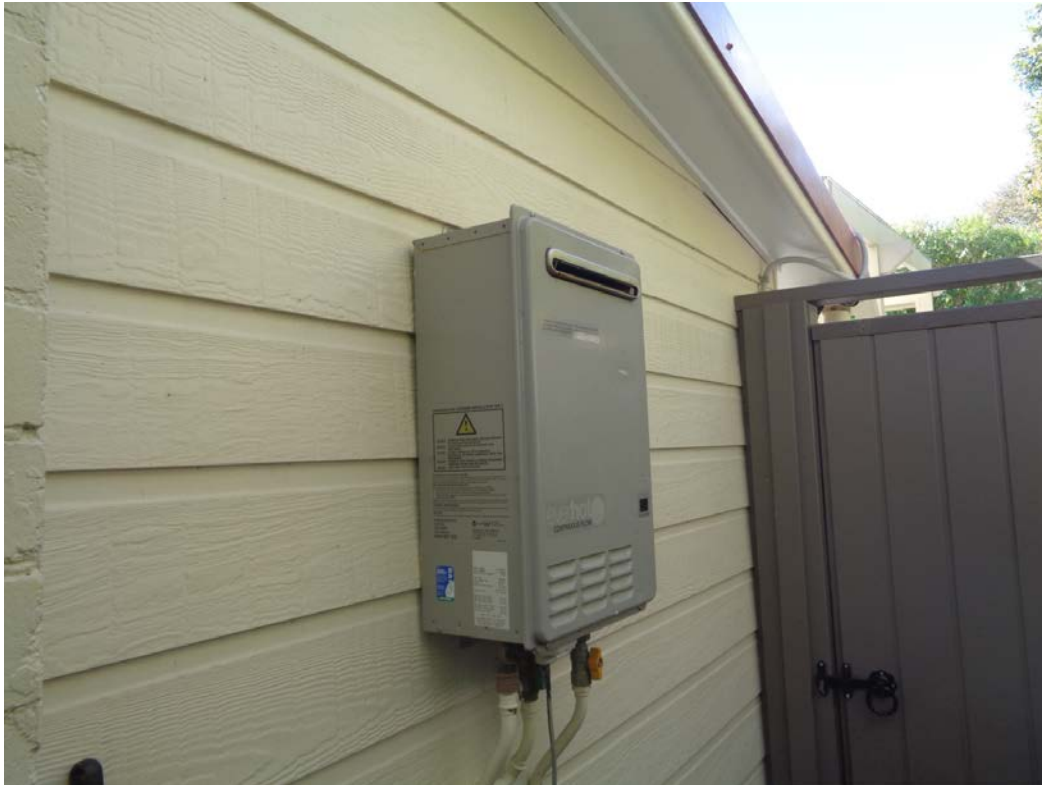
Gas hot water system
